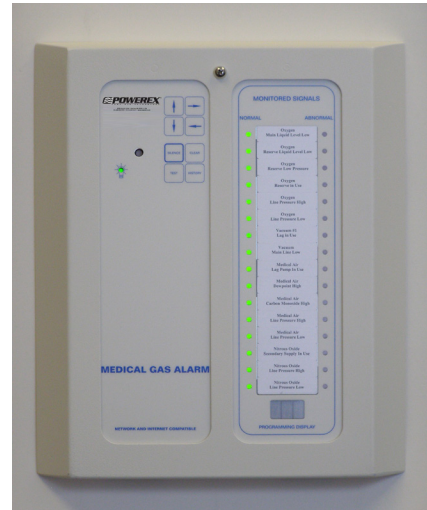
Master alarm shown above is 16 signals – part # PX-DU16
